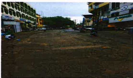
Present state of Nellikai road.
